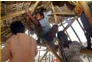
Children assist in the repair of a bamboo roof of a house damaged by the tsunami in India.
